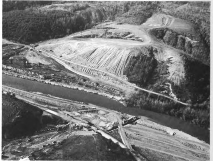
W. Kerr Scott Dam and Reservoir. This sequence of photographs follows the construction from site preparation to completion.
