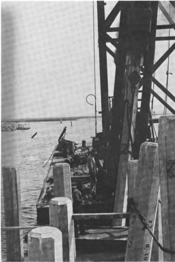
Reconstruction of the warehouse and wharf at the Ordnance Depot on the Cooper River, Charleston, in 1941. Scenes show the old dock and dock shed and the reinforced concret piles in the replacement structure.
