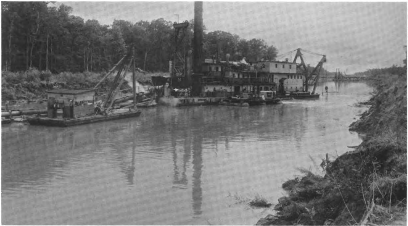
The dredges Tampa and Margate dredging in the intracoastal waterway section in back of Myrtle Beach, South Carolina in 1935.
