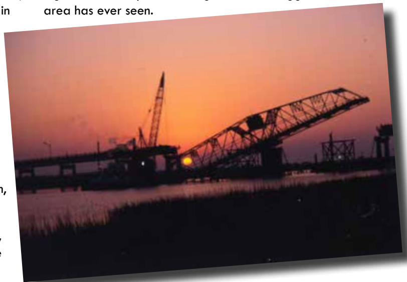
Left: The Ben Sawyer Bridge is seen tipped into the water as crews attempt to raise it after Hurricane Hugo. Photo from Charleston District archives Right: Nelson holds a photo of the bridge that he keeps in his home as a reminder of his work. Photo by Sara Corbett
