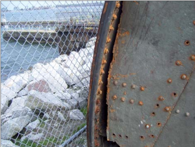
The old, rusted Tainter valve was starting to separate on the sides.
